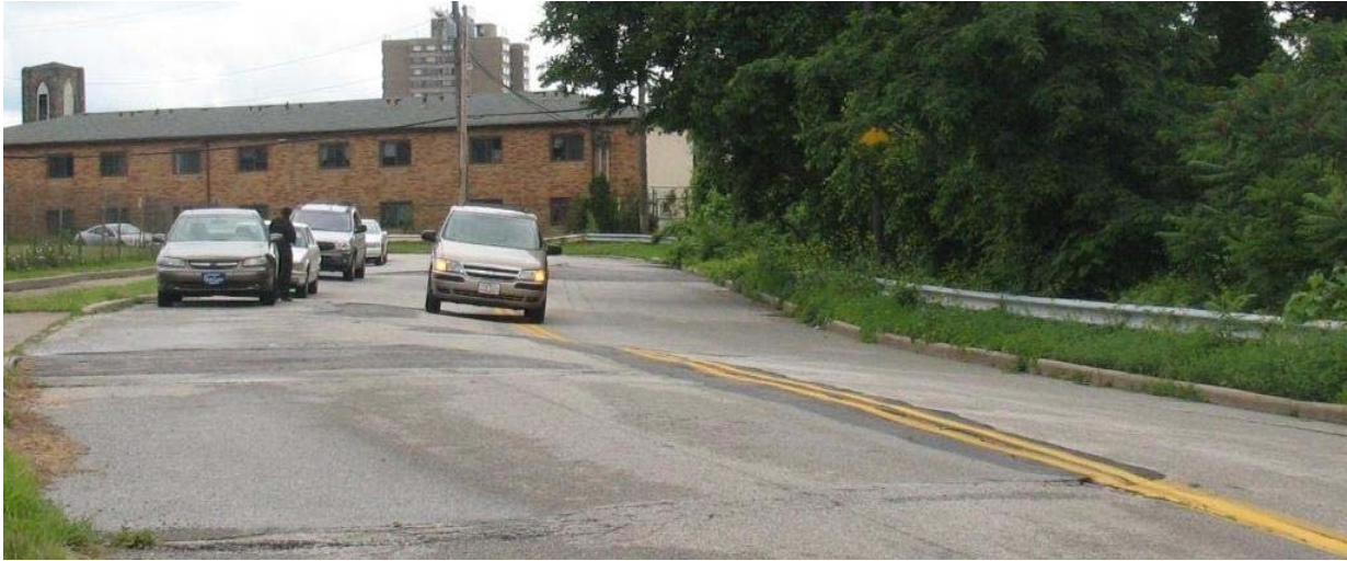
Image 6.1.7: Upper Slope Scarp Failure along Franklin Ave. Source: USACE Field Inspection, 30 Jun 2008
