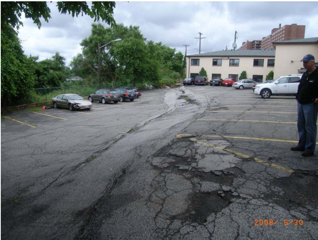
Image 6.1.8: Upper Slope Scarp Failure in parking lot along West 25 th Street. Source: USACE Field Inspection, 30 Jun 2008
