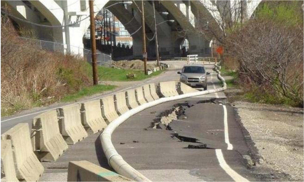
Image 6.1.2.: Riverbed St., Downstream Failure. Source: USACE Field Inspection, 19 Apr 2006
