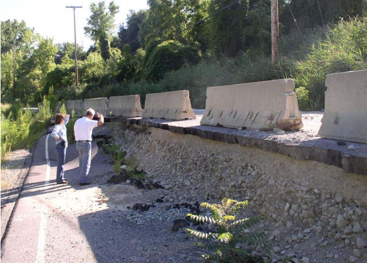
Image 6.1.4: Riverbed St., Downstream Failure. Source: USACE Field Inspection, 20 Aug 2008
