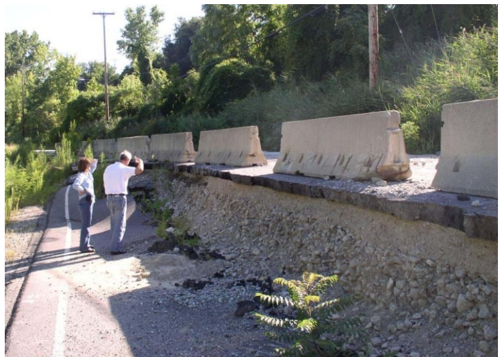
Riverbed St., Downstream Failure. Source: USACE Field Inspection, 20 Aug 2008
