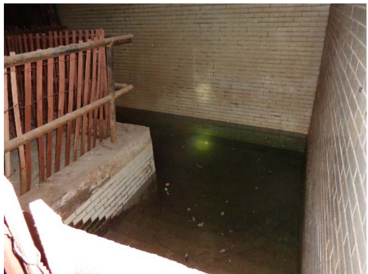
Figure 7: Bypass Tunnel Flooded with Water
