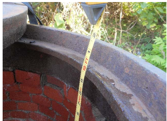
Figure 15: Water Depth in Partially Plugged Manhole
