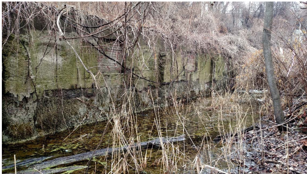
Figure 20: Lederer Building Foundation (Trapping Water)
