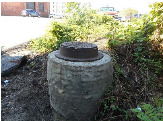
Figure 14: Partially Plugged Manhole as shown in Figure 11
