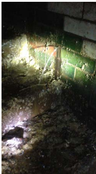
Figure 12: Water Penetrating through Walls
