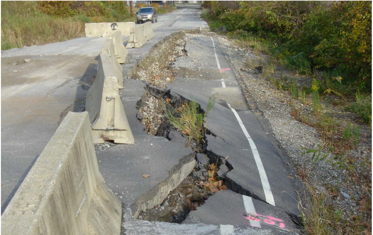
Image 6.1.3: Riverbed St., Downstream Failure. Source: USACE Field Inspection, 19 Nov 2007
