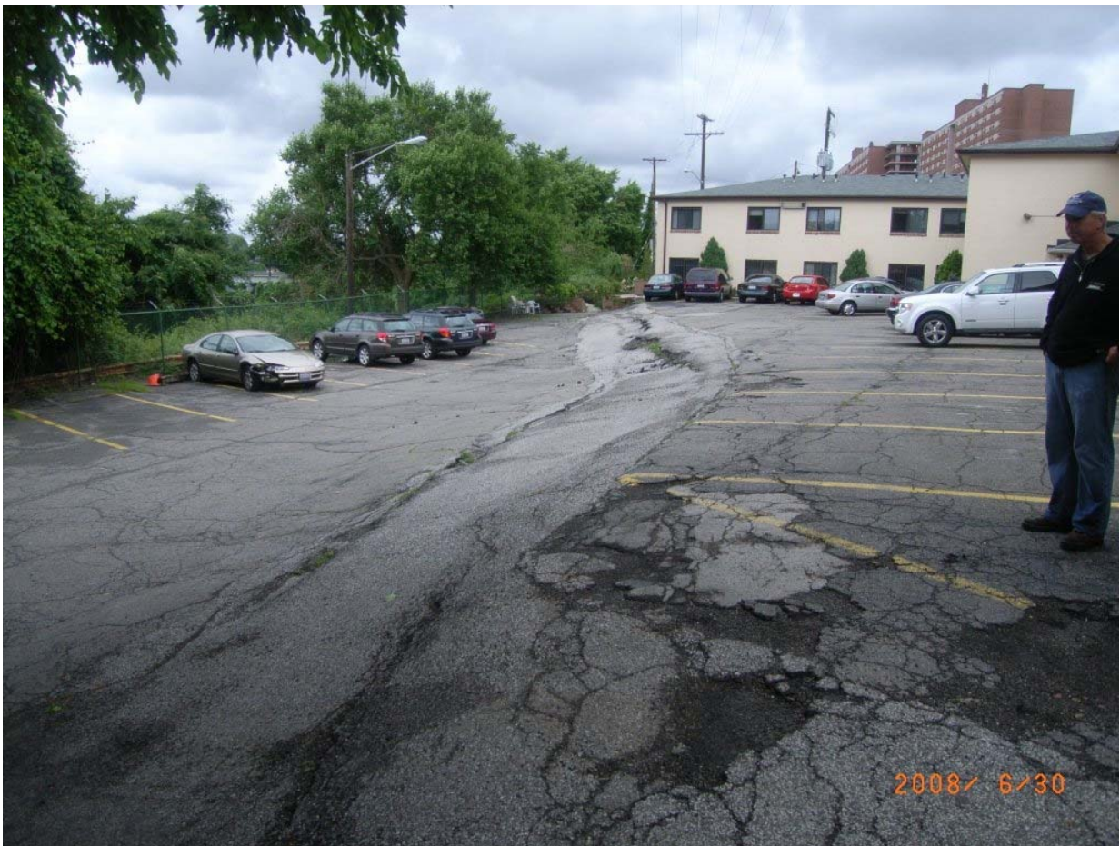
Image 6.1.8: Upper Slope Scarp Failure in parking lot along West 25 th Street. Source: USACE Field Inspection, 30 Jun 2008
