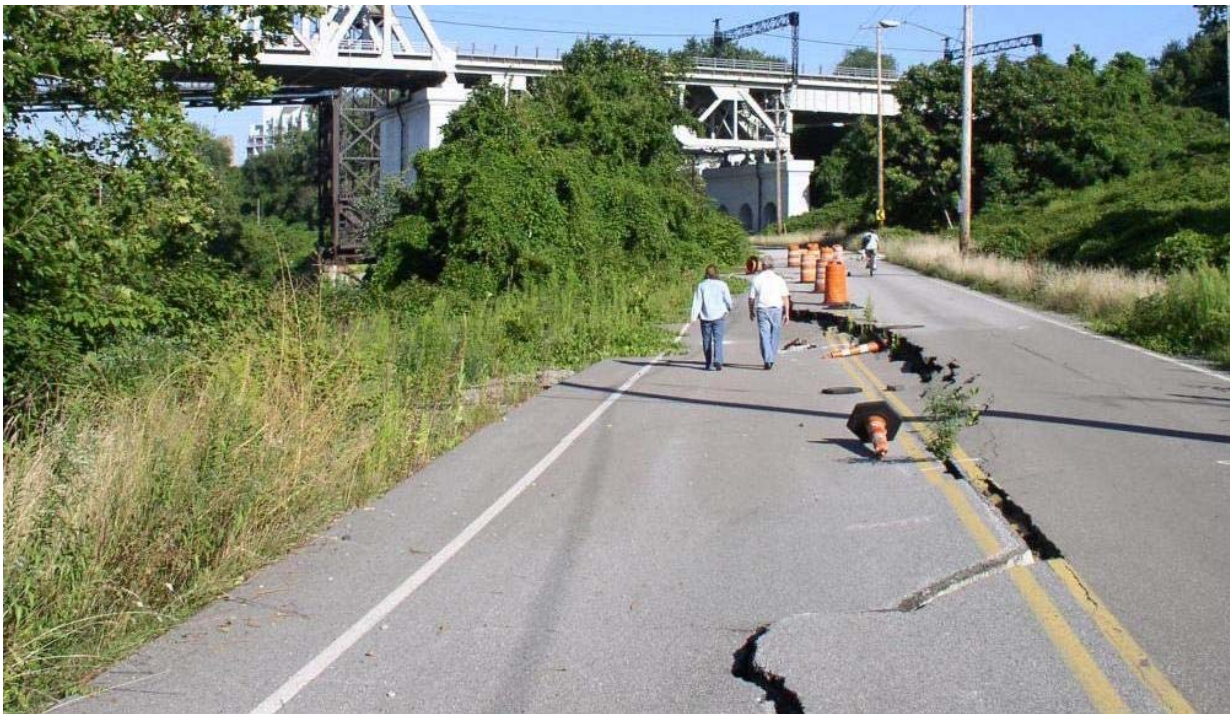
Image 6.1.6: Riverbed Street, Upstream Failure. Source: USACE Field Inspection, 20 Aug 2008
