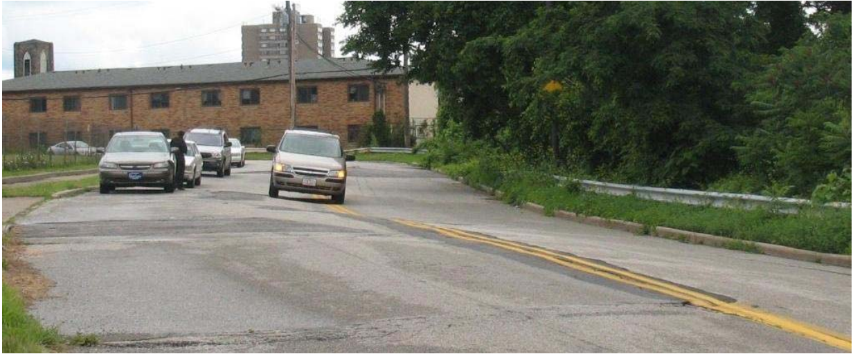
Image 6.1.7: Upper Slope Scarp Failure along Franklin Ave. Source: USACE Field Inspection, 30 Jun 2008
