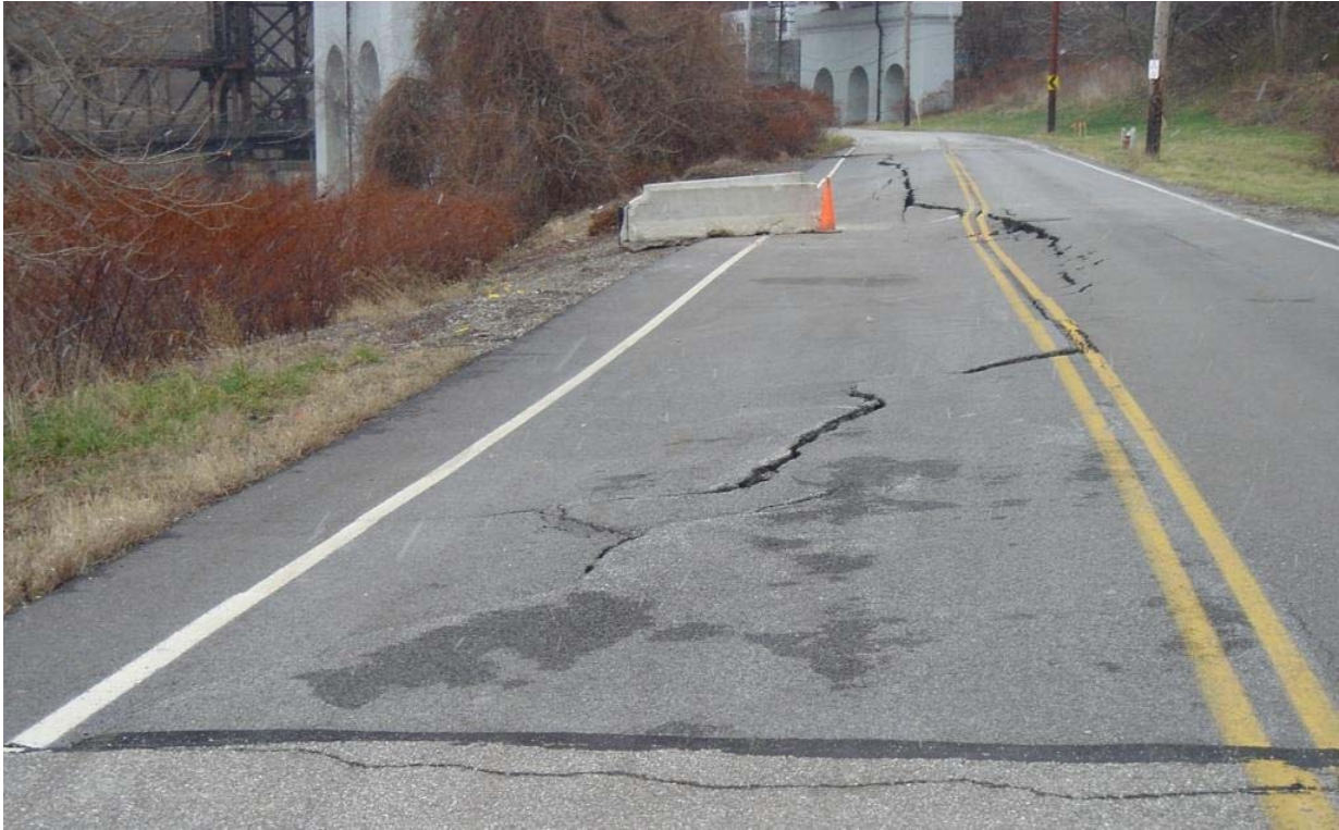
Image 6.1.5: Riverbed St., Upstream Failure. Source: USACE Field Inspection, 8 Jan 2007
